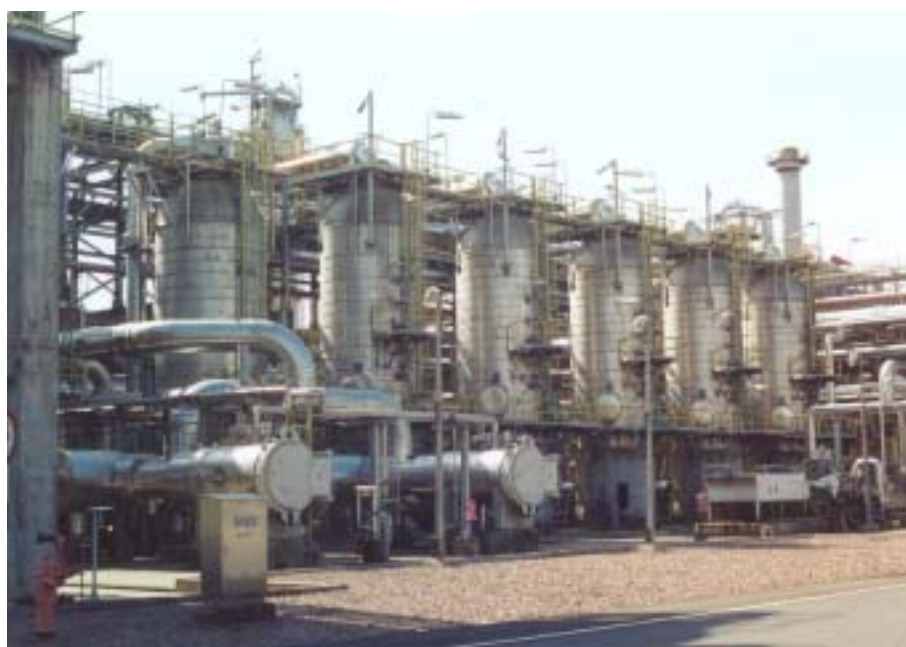
Natural Gas Drying Unit
